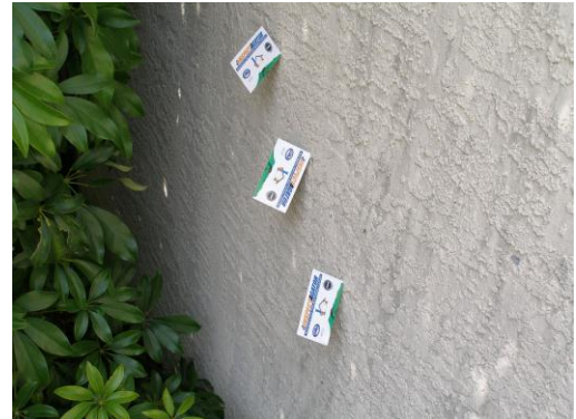
If I can "slip" my business cards in the cracks, how hard do you think it is for water to "slip" in?
